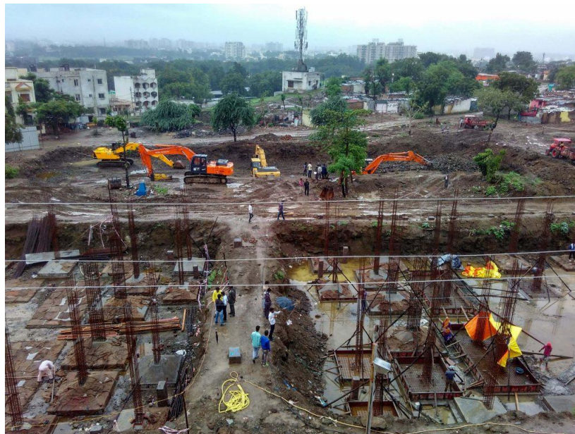
Fig -1: An under construction slum relocation site for Pradhan mantra Awas Yojana at Bhuri Tekri in Indore
