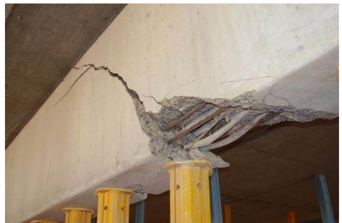
Fig - 2 : Shear Failure in RCC Beam
