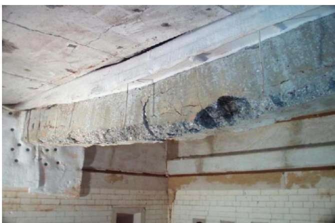
Fig -1 : Flexural Failure in RCC Beam
