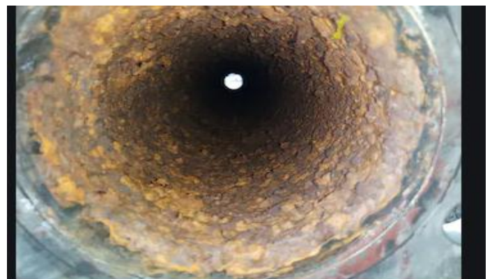
Fig -2: Corrosion in Pipes
