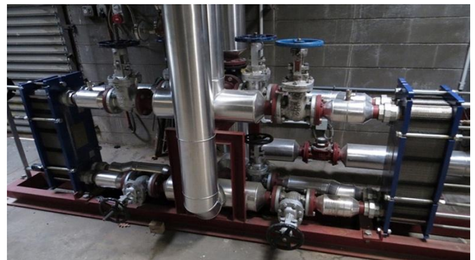
Fig 3: Primary heat exchanger and valve
