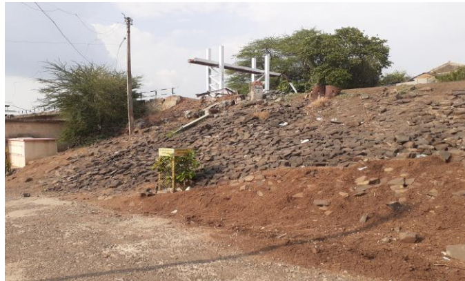
Fig 1.7 Erosion of side slope of road
