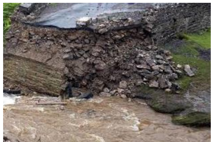
Fig. 1.5 Slope failures due to hammering of flood water
