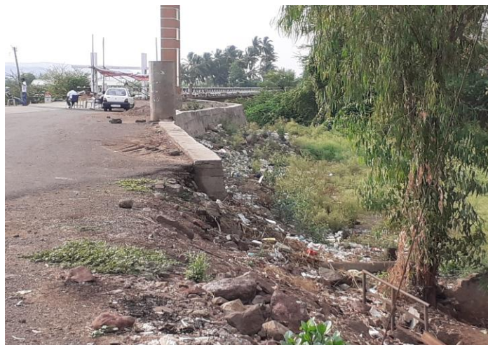
Fig. 1.8 Side slope failure of road belongs to Krushna Bridge
