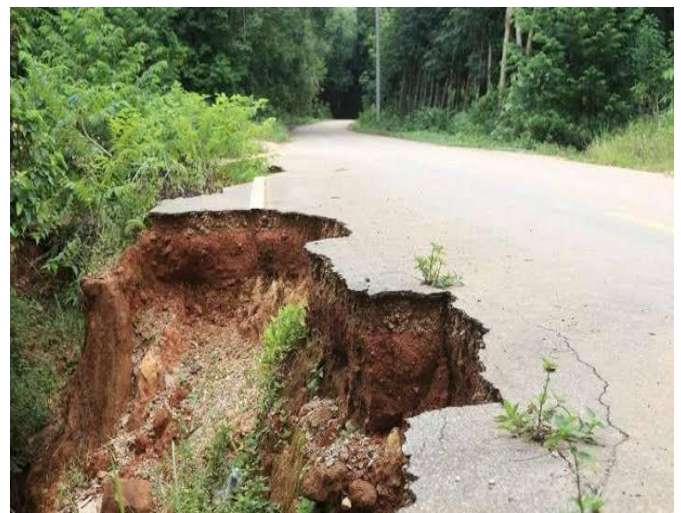
Fig 1.6 slope failure at side of road
