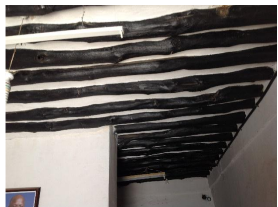
Figure 15: Mangrove poles to Support Upper Floors and Ceiling Below of the Bagamoyo Fort Source: August 2019 Field Survey
