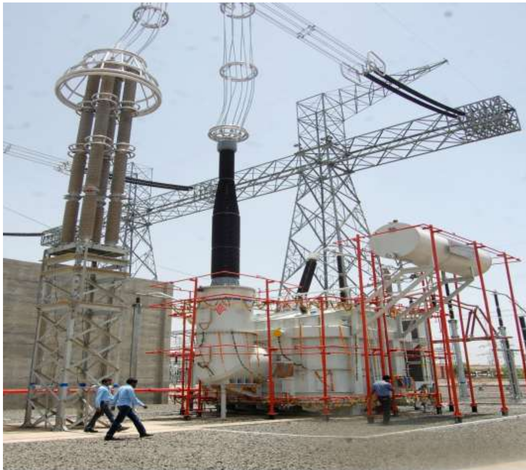
World's Highest Voltage Transformer 1550/400/33 kV at our Bina S/s (Central India)
