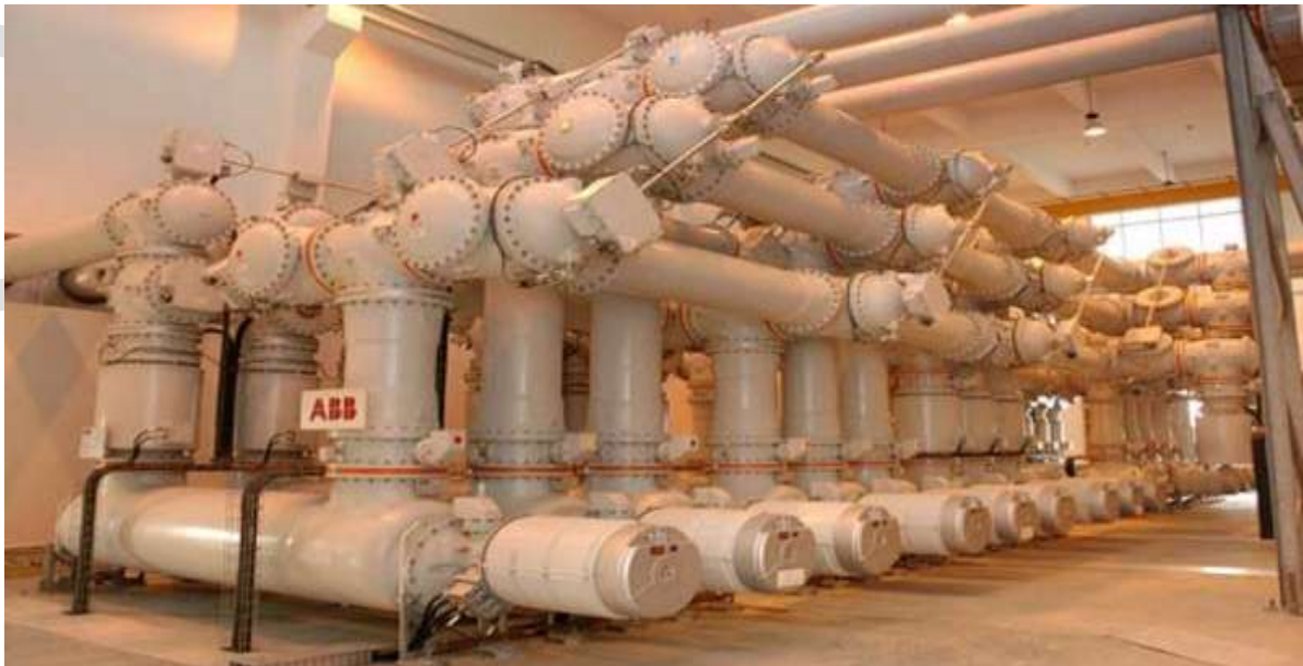
Fig.4:Gas Insulated Substation ( Source- Power Grid )
