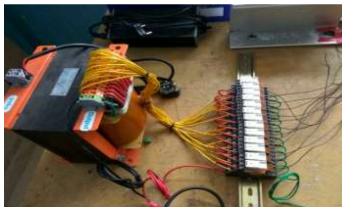
Fig-2: Tap converting transformer connected with relays.
