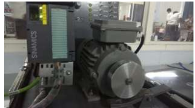
Fig 7: Running of Motor at controllable speed
