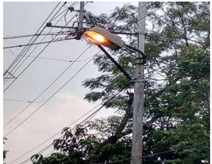
Fig-2. Street Light Still On In Morning
