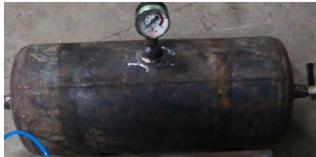
5.3 compressed air tank
