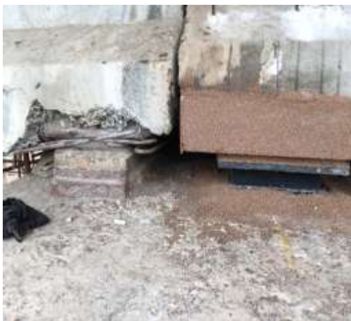
Fig 4. Deteriorated old bearing and newly replaced bearing.
