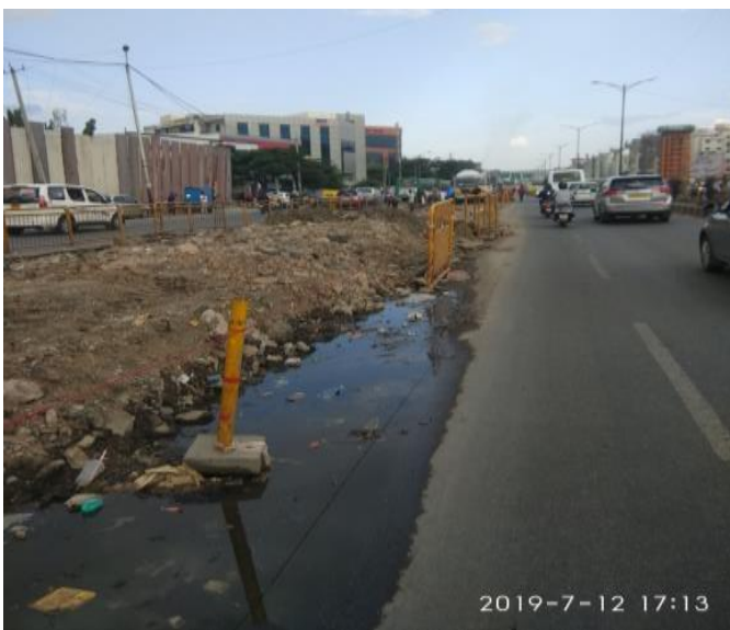
Fig -1: IMPROPER MAINTENANCE OF ROAD SIDE DRAIN AT BLACKSPOT 1
