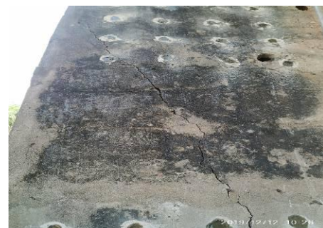
Fig -2: Major cracks observed in abutment
