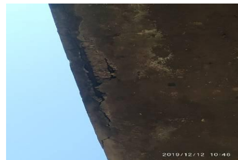
Fig -1: Reinforcement exposed, corrosion, cracks observed in slab
