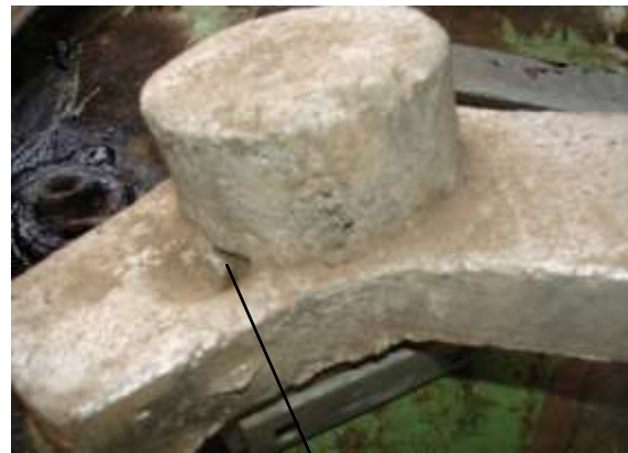
d) Shrinkage at the joint of section
