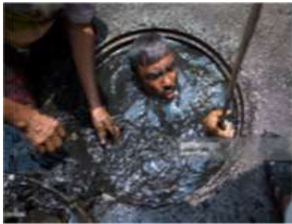
Fig 1a: Manual scavenger clearing blockage in a manhole
