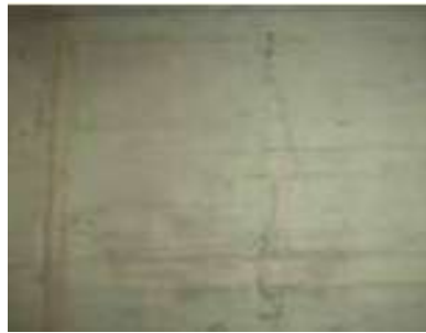
Figure No. 4 Drying Shrinkage cracking
