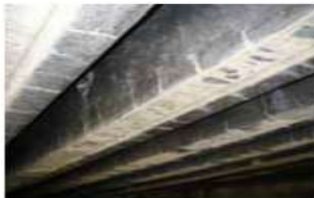
Figure No. 2 Flexural cracks that self sealed through autogenous healing
