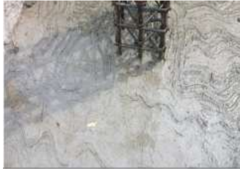
Figure No. 3 Plastic Shrinkage cracks
