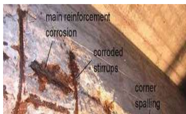
Figure No. 5 Longitudinal cracks at corners of crosshead associated with corrosion of steel reinforcement
