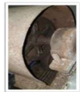
Figure 11: No lubrication done for gears
