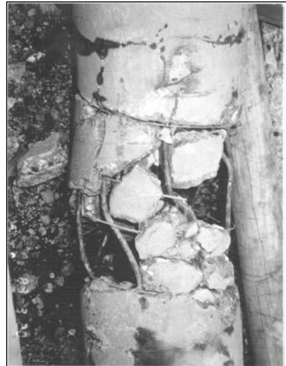
Fig-3: Damage to pile by 2m of lateral ground displacement during 1964 Niigata earthquake (Yoshida et al. 1990)
