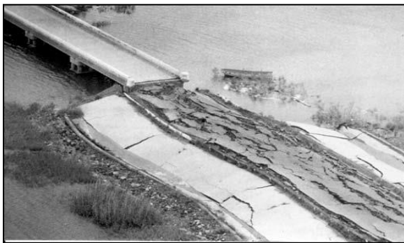
Fig- 4: Bridge on undamaged pile foundations with failed approaches due to liquefaction (Finn and Fujita 2002)
