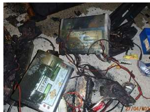
Fig -3: Lithium ion battery destroyed due to fire
