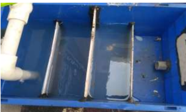
Fig 4 Shows settling chamber and baffle walls
