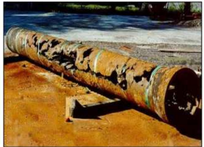
Figure 5. completely corroded pipeline.
