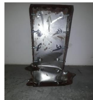
Fig 13: Failure of bolted column
