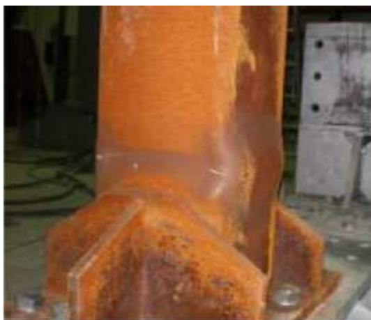
Fig -8: Failure Mechanism during Cyclic Test
