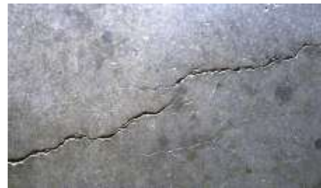
Fig No: 4 Crack Defect
