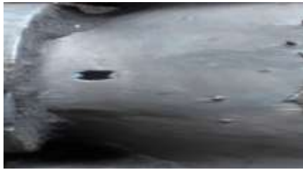
Fig No: 2 Cold Shut
