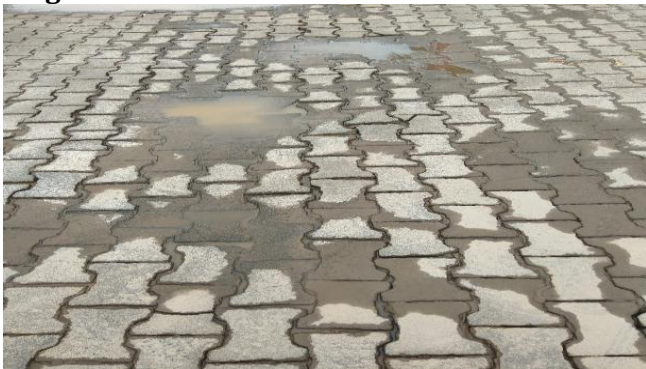
Fig-1: Pavers uneven and sitting at different heights
