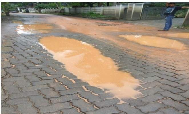
Fig -2: Water puddling on pavers
