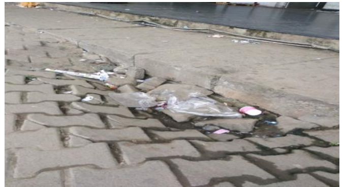
Fig-3: Border pavers are falling off
