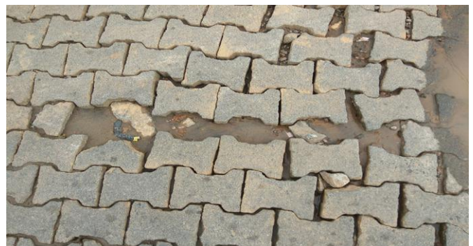
Fig -4 : Individual pavers separating
