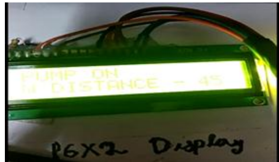
Fig. 5.2 Output: Pump On
