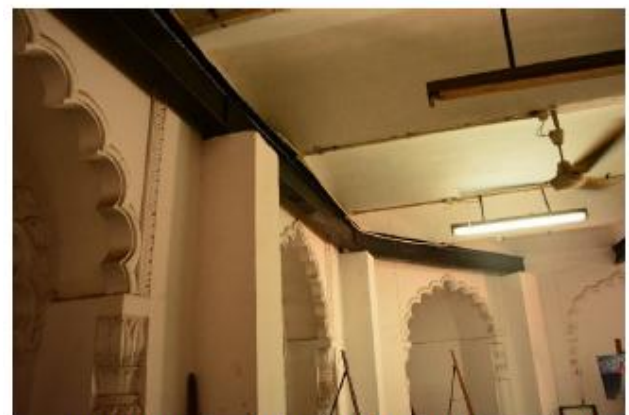
Arches and columns transferring the load to the ground at the ends.
