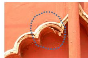
Damage of Decorative work
