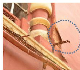
External wall are about to lose its lime plaster
