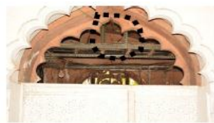
Suspended cables to the ceiling
