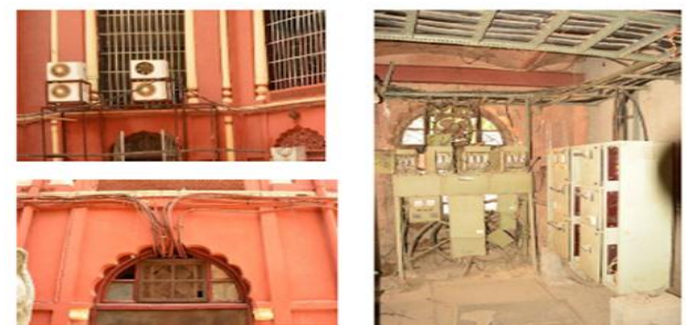
Various electrical services have been inserted into the building in an appropriate manner disturbing the visual aesthetics of the building.
