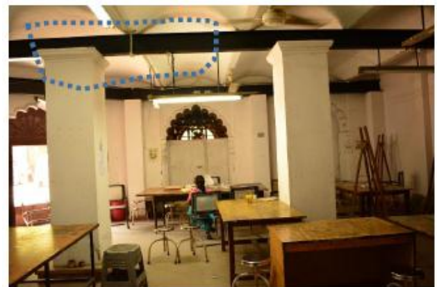
I-section running through each end of vaults finally transferring the load to the columns
