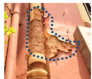
Flaking & Peeling of plaster
