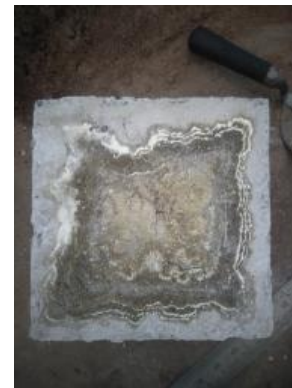
Fig -7.4.3: Acid Reaction of concrete
