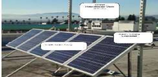
Fig. 6. The experimental setup for the grid voltage and current measurement.
