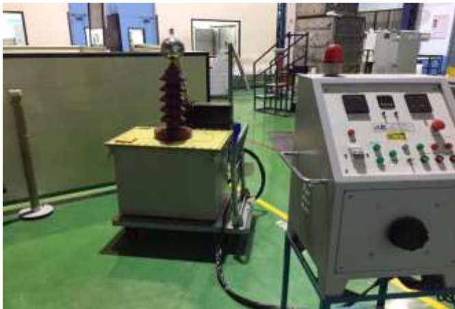
Fig. Auto Earth System for HV test set up.
