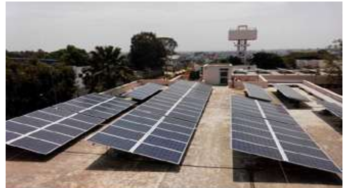
Fig-3: Mono Crystalline PV Panels
