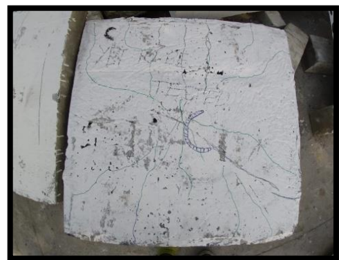
Fig - 10: Crack pattern on conventional slab
