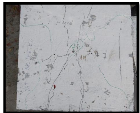
Fig - 11: Crack pattern on uniform arrangement
