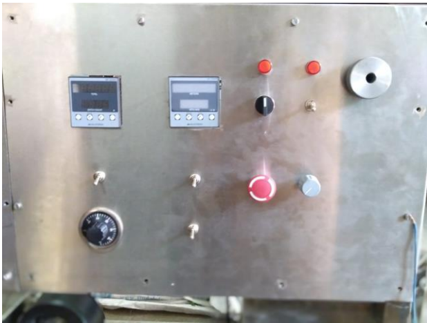
Fig.7. Control panel of LNM
