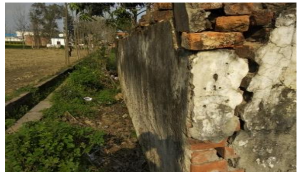
Fig 4- Wall with empty joints
