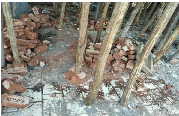
Fig 2- Loose brick support
