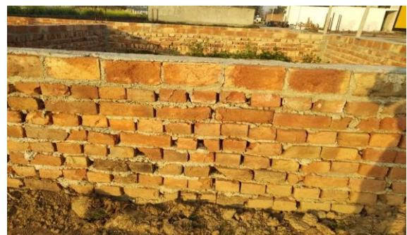
Fig 5- Wall with bonding cracks
