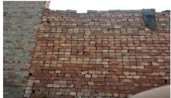
Fig 3- Brick wall with no mortar
