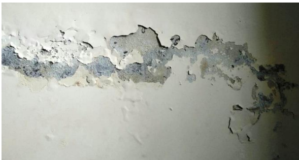
Fig 6- Moisture Patches on wall
