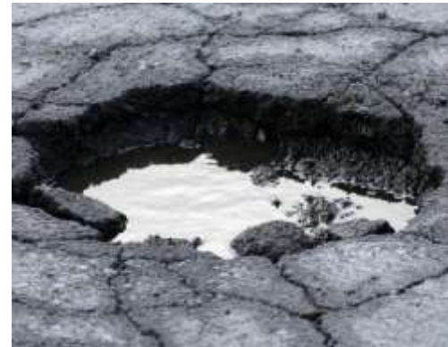
Fig. 1. Condition of roads with potholes
