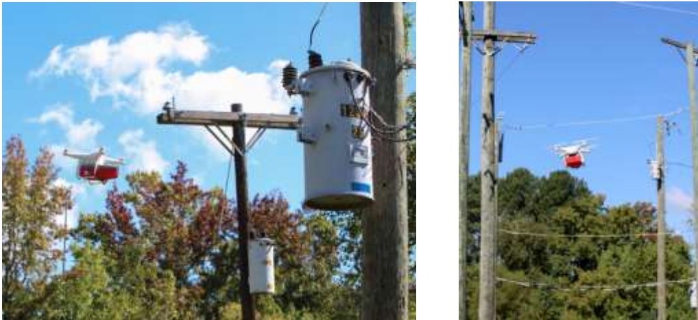
Fig. 5. Drones navigating electric grid components.
