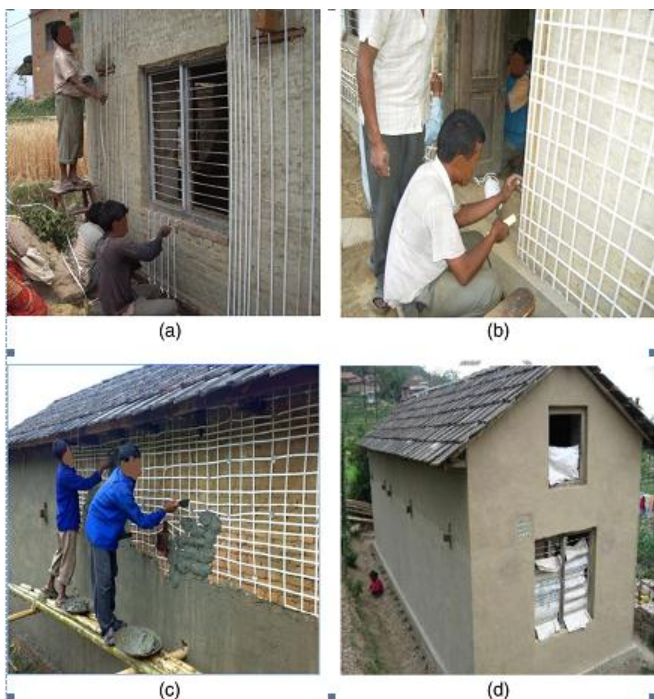
Fig. 9: Different stages of reinforcing the masonry building with PP band: (a) wrapping near window; (b) wrapping near door; (c) plastering after wrapping; and (d) completed PP band-retrofitted building
