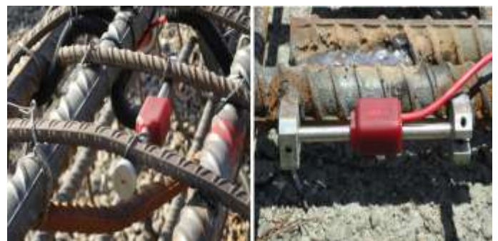
Figure 31: Vibrating wire gauges used in rebar to monitor strain [106]
