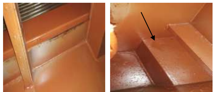
Fig -8: (1) Cooler side: oil not found (2) Side portion of NDE Bearing: Few drops of oil found
