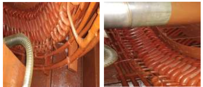
Fig -5: Bottom side of NDE bearing: Minor oil seepage observed
