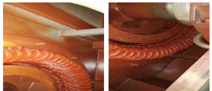
Fig -7: Overhang winding: No oil observed in both side of winding
