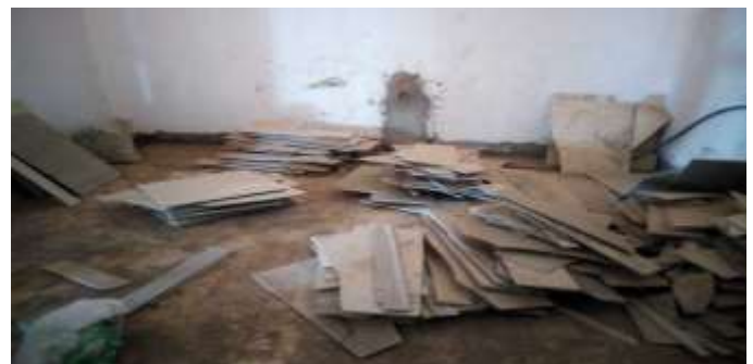
Fig 9: Wrong storage of ceramic
