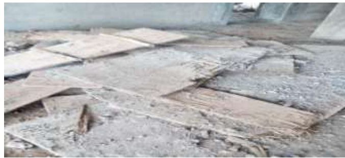
Fig 11: Wastages of formwork due to wrong fixing and dismantling
