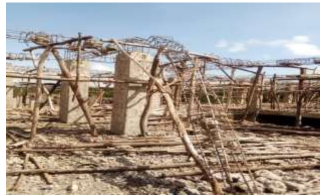
Fig 10: Wastage of during demolition
