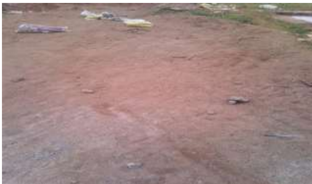
Fig 8: Poor handling/ management of sand on site
