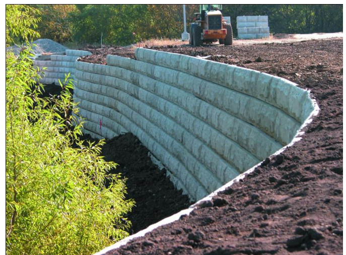
Fig -5: MSE Wall used for Slope Protection
