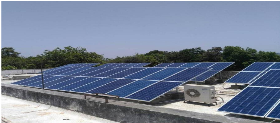
Figure : 15 kw power plant in Jaipur city.
