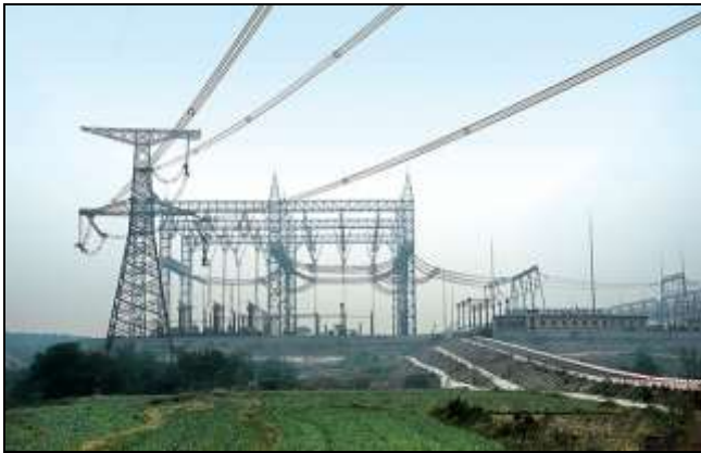
Figure-3. Intelligent Substations (China)
