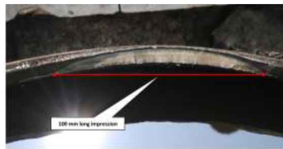
Figure 4a: Rupture at longitudinal pipe seam
