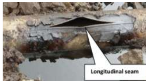
Figure 3b: Preliminary failure photographs at site
