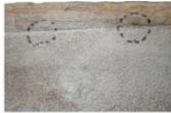
Figure 5a: Weld defects visible in HAZ& weld zone
