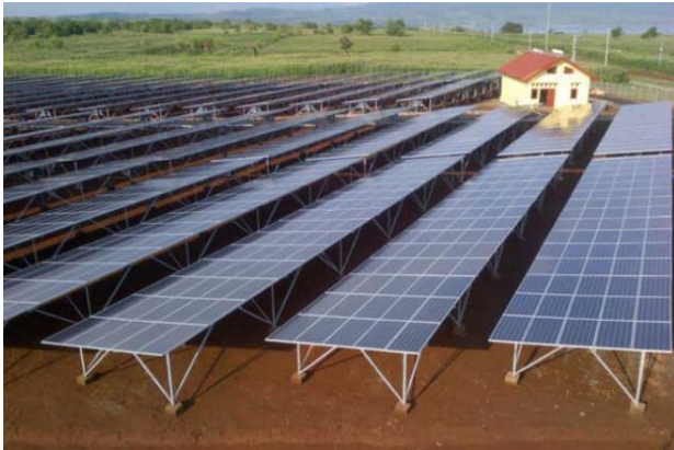
Fig 9: 1 MW grid connected solar PV power plant
