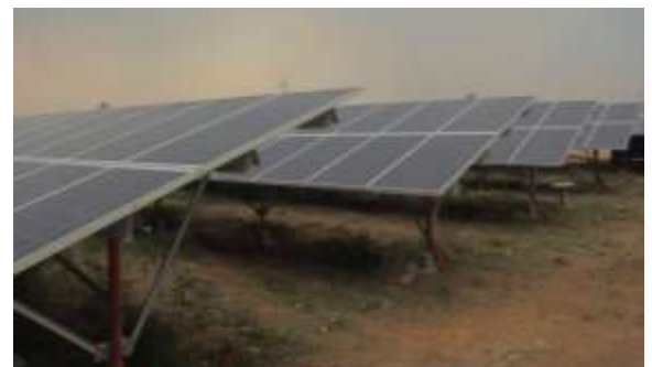
Fig-2: Solar PV modules placed on mounting structure
