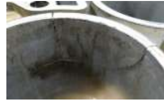
Fig -3: Liner installation failures finally, one of the most bizarre failures.
