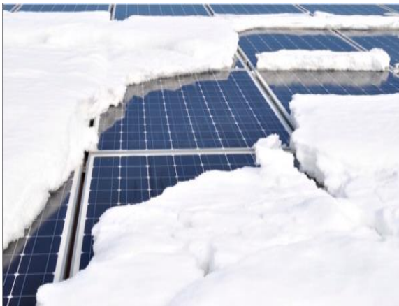
Fig-1: Solar Panel works on Antarctica even covered with ice partly.
