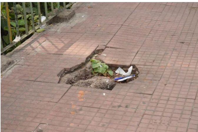
Fig -3: Damages of flooring on foot path
