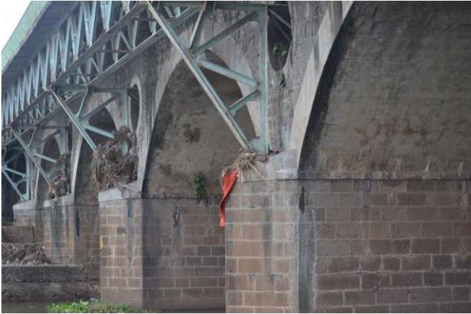
Fig -2: Rubbish Stuck in the Steel Truss
